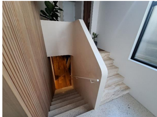
Figure 6: 9B stair to unauthorised basement.
