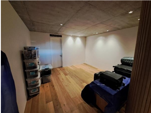
Figure 3: 9A unauthorised basement.
