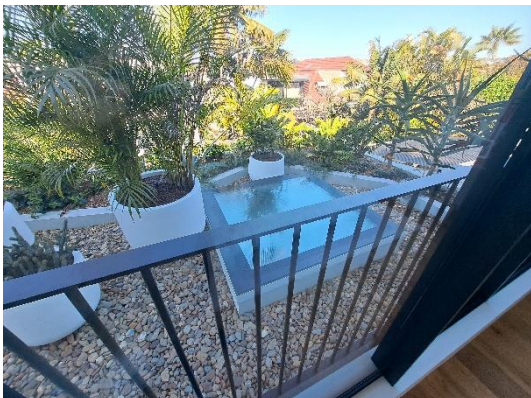
Figure 7: 9A unauthorised skylight.
