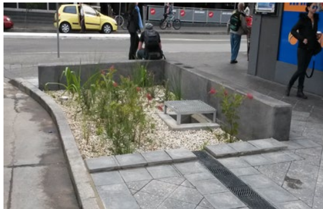
Bioretention Raingarden at Gray Street North
