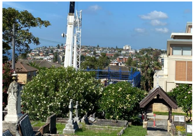
Figure 2: The current construction and scaffolding on site viewed from South Head Road Cemetery.
