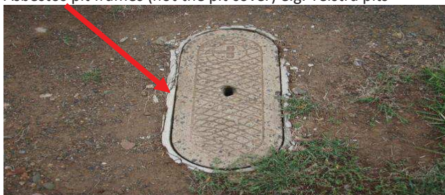
Asbestos pit frames (not the pit cover) e.g. Telstra pits
