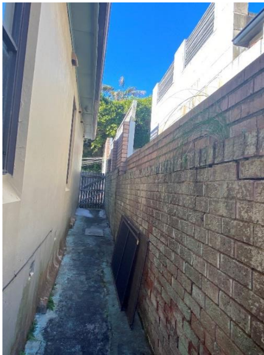
Figure 4: Existing southern side setback, looking east towards rear yard of subject site.
