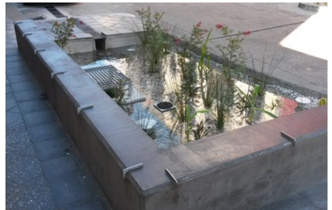
Newly constructed bioretention raingarden at Gray Street North
